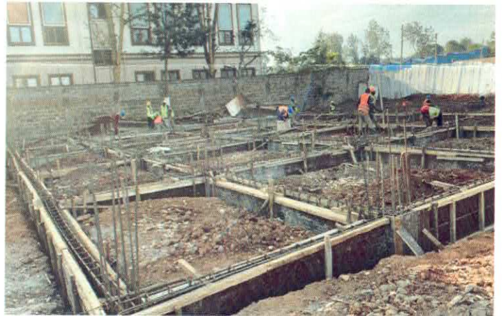
September 2024, Foundation work for the new facilities to house Runda Baptist Church.
